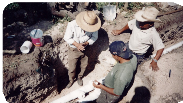
New pipeline near San Lucas Tolimán, Guatemala. The role of local government in public works on private or public land varies considerably around the world. (photo: S. Furey)
