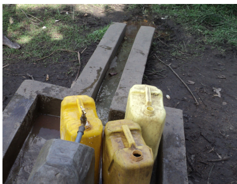
A tapstand in Kabarole district. Piped schemes provide quality water for people
