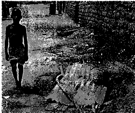
Badly constructed soakaway pits for domestic wastewater
