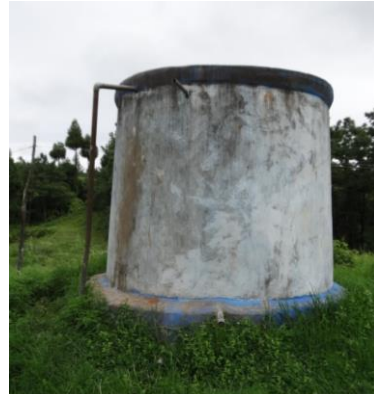
Storage tank at Mawklot and in Umylympung
