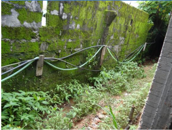
Poly pipes carrying water from private springs
