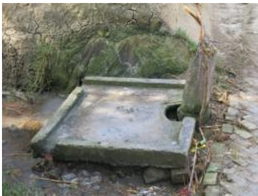
Photo 5: Broken tap-stand of the piped supply system in Dakshin para
