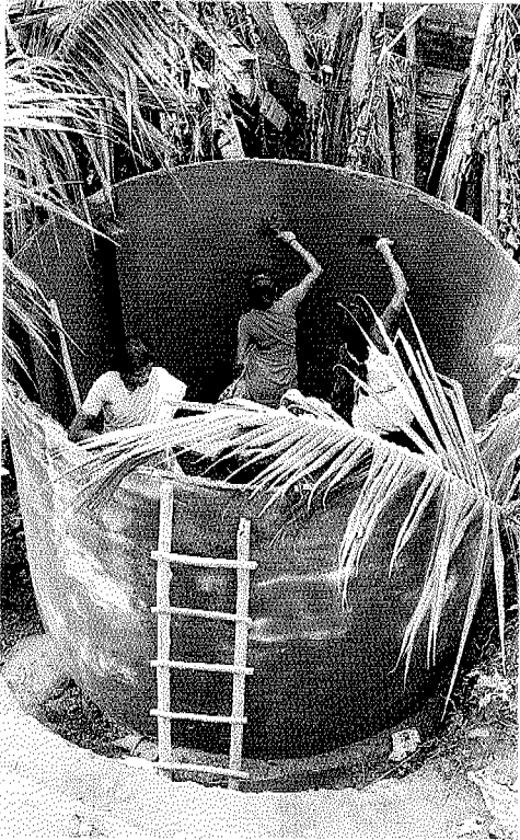
These Tamil Nadu women masons are constructing a ferro-cement rainwater harvesting tank.
