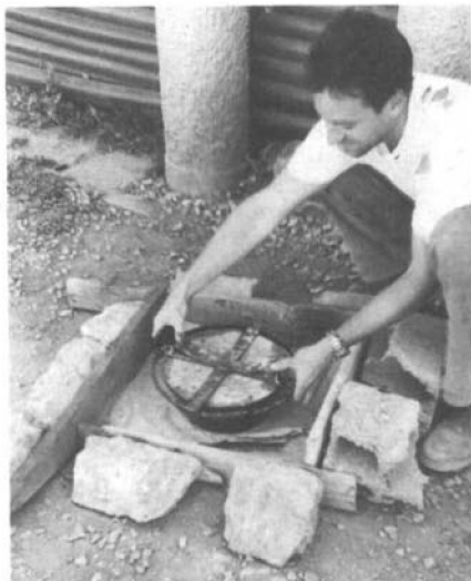
Figure 2. A fixture attached to the mould can be used to produce the lip.
