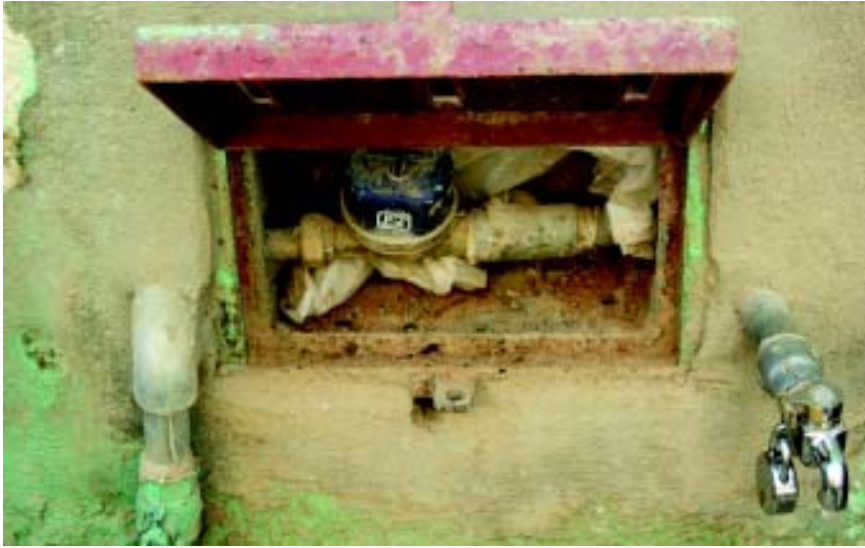
A newly-installed meter and outside tap locked by the household for private use.
