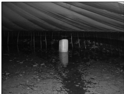
Scum on the surface of the water affects the turbidity of the treated water. The jerry can supporting the floating outlet is also shown.
