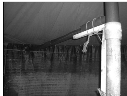
The scum collector pipe is fixed onto the tank roof support and overflow outlet.
