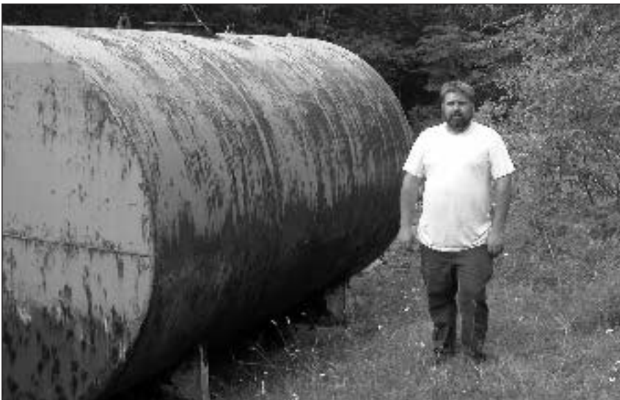
The water operator for Whitmer, West Virginia (population 150), stands next to the ageing town water tank. The Rural Community Assistance Program has helped the community to organize, finance and install upgrades to the town's water system
