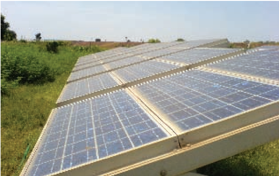
Solar panels for a small piped water scheme in the region of Kayes in Mali
