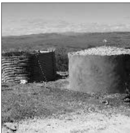
A new water tank, and one in the process of being constructed
