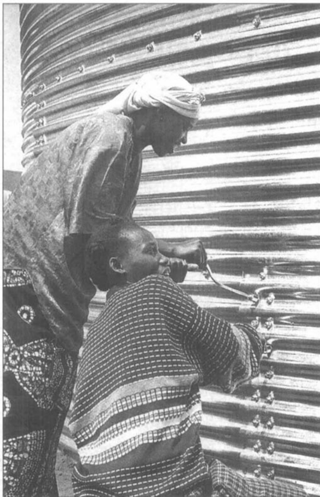
Women build an Oxfam tank in the Goma camp of Mugunga, August 1994.
