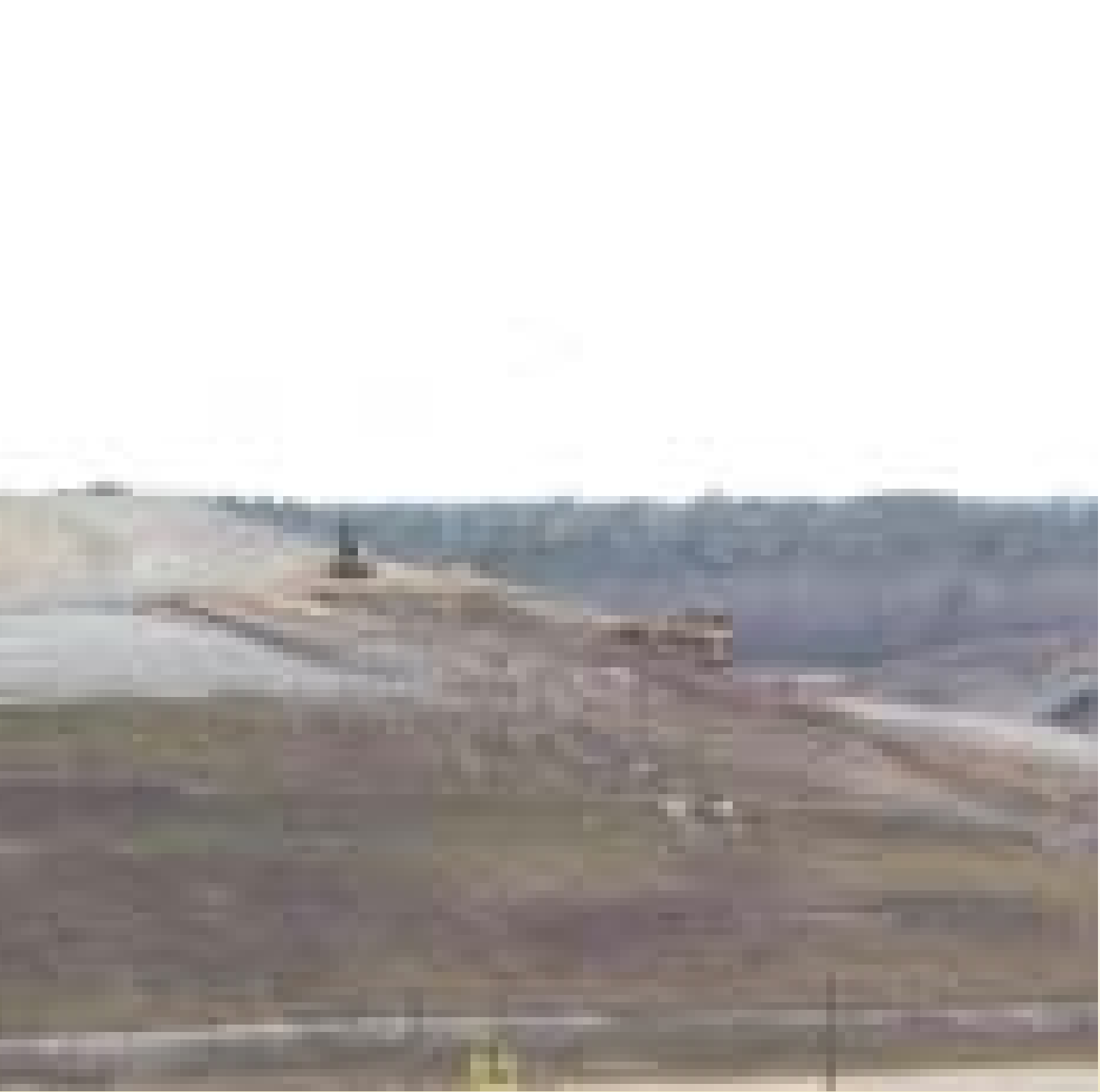
Waste being compacted after dumping, Jones Cross Roads Landfill Site, Delaware, USA.
