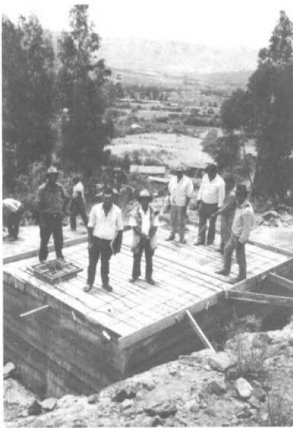
This water storage tank will be part of a system serving a community of 500 people.
