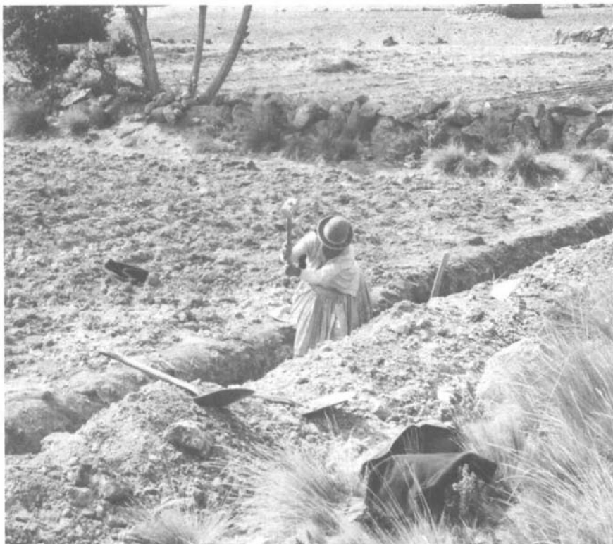
Unpaid community labour is used to dig the several kilometres of trenches needed for each system.
