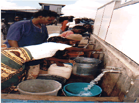
Figure 3-6: Communal Standpipes in George Township
