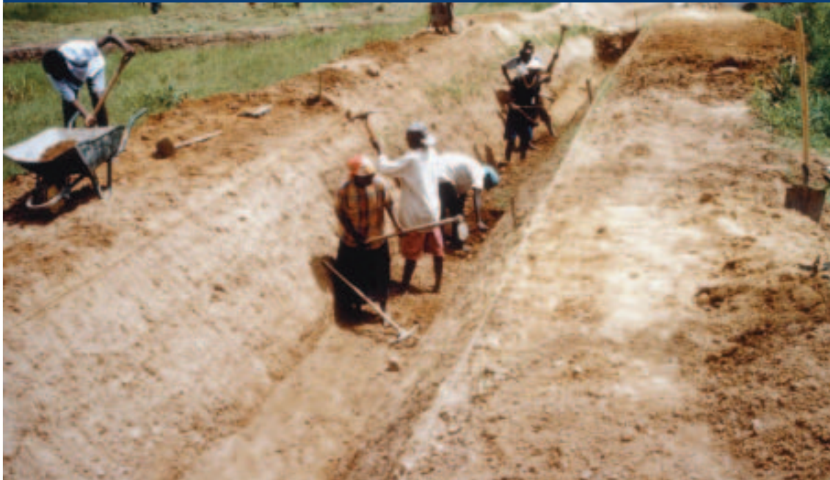
Plate 4 Section of the left bank of the principle canal under construction at Bishenyi (Rwanda)
