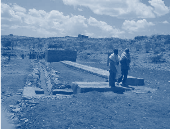
Figure 3.16. Filtration gallery for drinking water (right) in the multi-purpose system in Adidaero, Ethiopia: the underground canal from the diversion dam splits into an irrigation canal (left) and the filtration gallery (photo: Eline Boelee)
