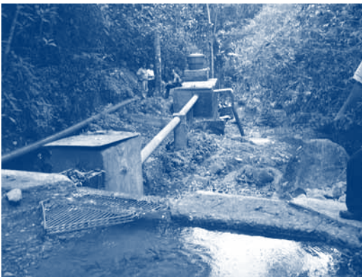
Figure 3.22. A multiplicity of pipes makes it difficult to monitor water intakes in the stream of the El Chocho catchment (photo: Grupo GIRH - Cinara)
