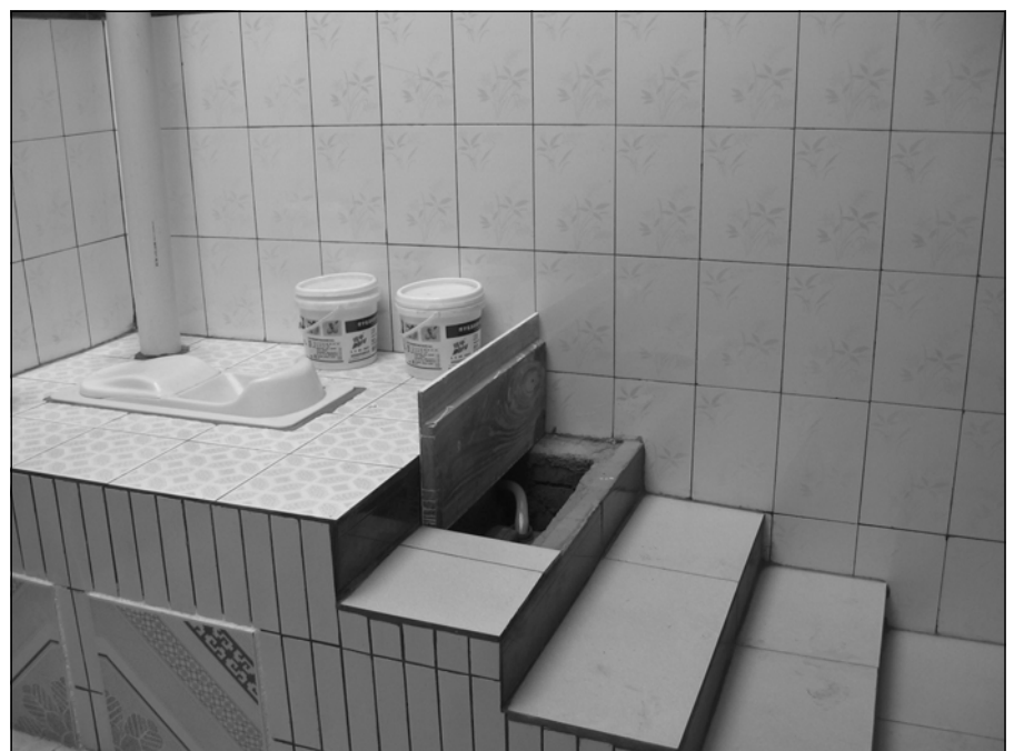
The urine-diverting toilet, showing position of the small urine-collection container and access to the two pits.
