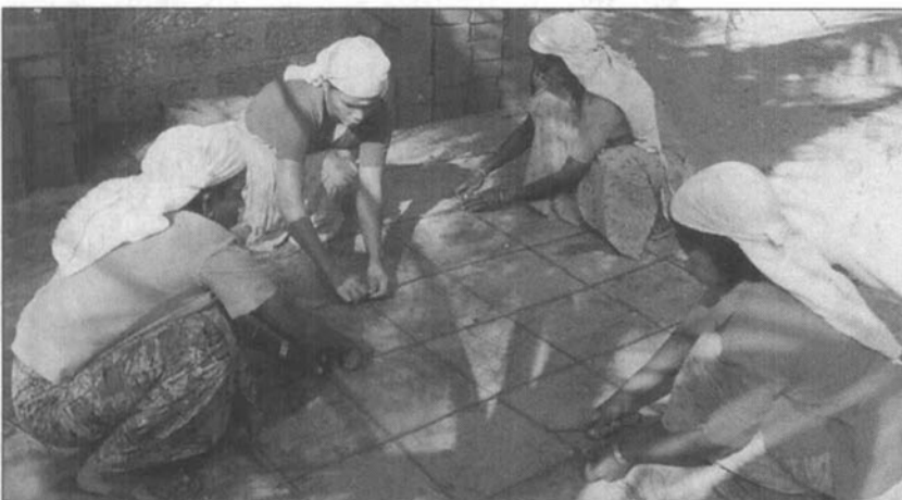
Training in progress — these JEEWOMS trainees are preparing steel for the roofs of latrines in construction.
