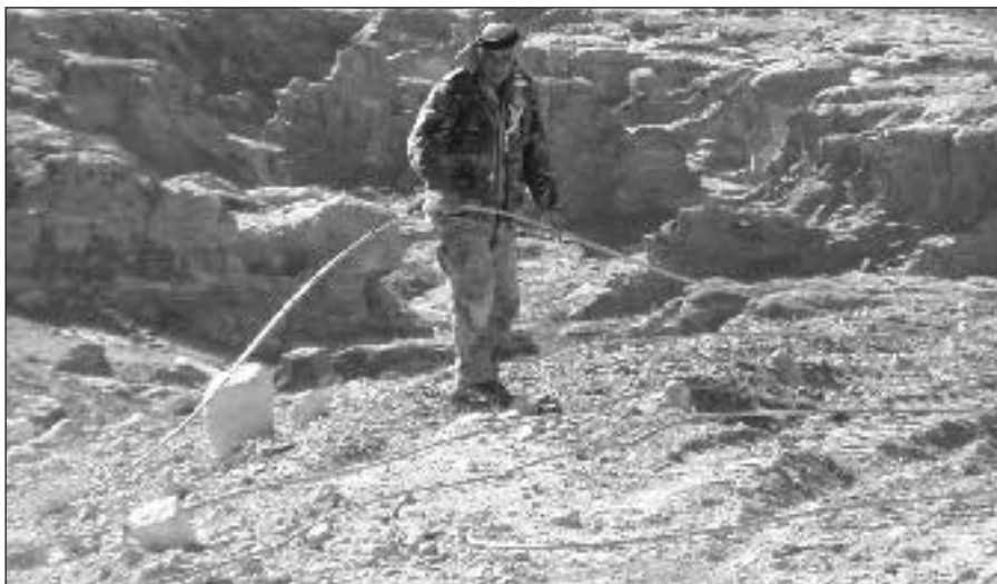
A community member lays locally manufactured colour-coded drip-lines for a pilot project in Wadi Musa, Jordan, providing reclaimed water for irrigation of tree crops, ornamentals and fodder.
