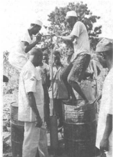
Hand-augering continues inside the PVC casing after the watertable has been reached.
