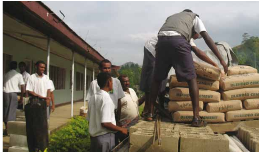
Project-based action: Action plans leading to the building of twenty handwashing basins in Sigatoka, Fiji
