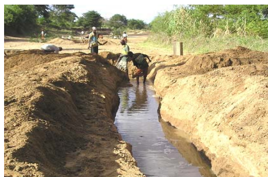
A flooded trench for infiltration pipes.
