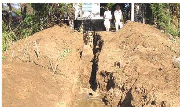
Infiltration pipe connecting to the intake.
