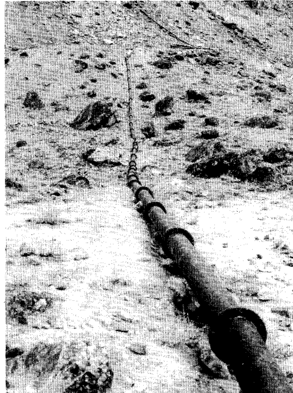
Old and new ideas combined. In Gilgit district, some villagers decided to build a 3,300-ft.-long inverted syphon out of flanged steel pipe.
