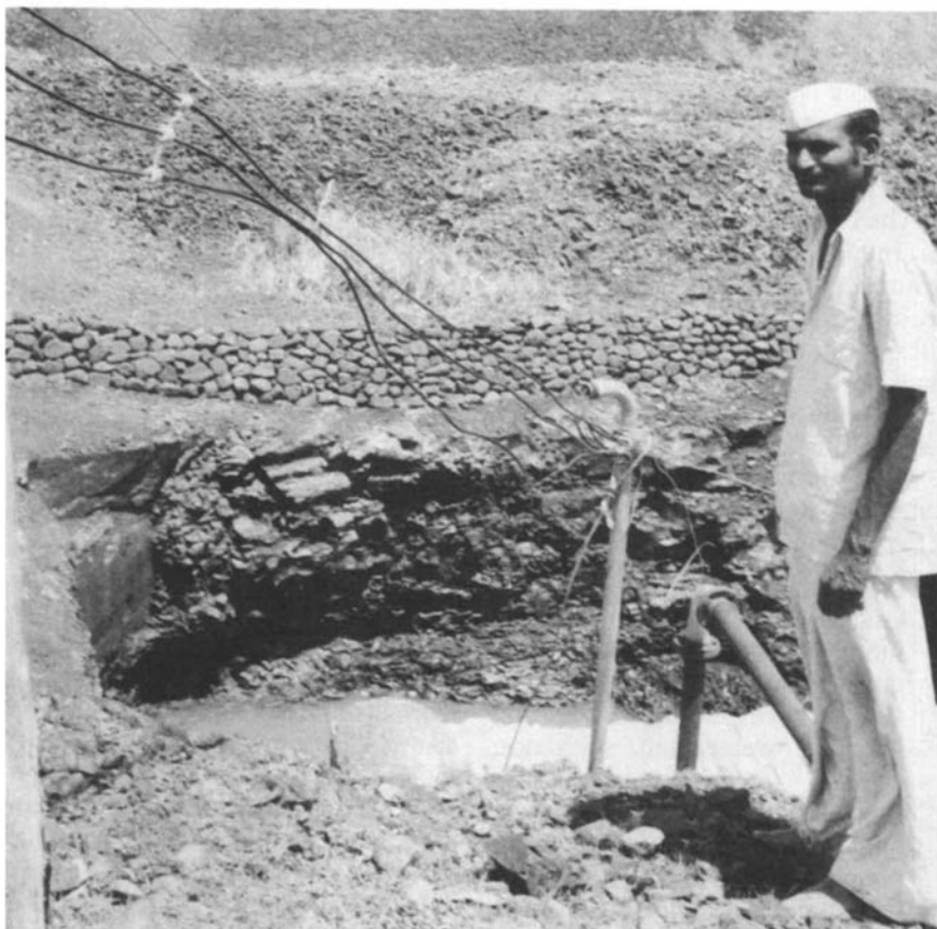
Progress was so good that they had installed three standpipes by 1983. The land irrigated in this scheme is luckily quite close to the pump. This work requires capital, and a unified community
