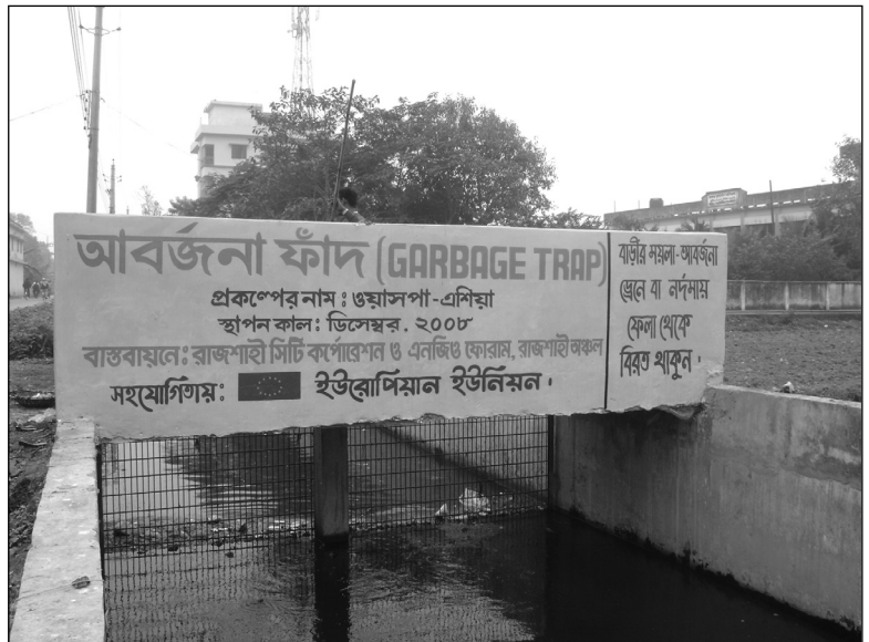
Garbage trap on the drain
