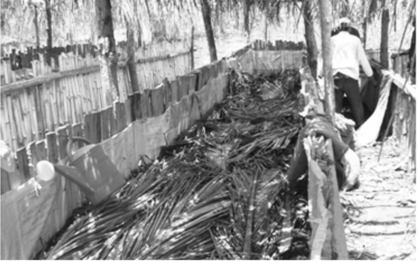
Photo 20: Construction of the vermi-compost need not be expensive and consist of local materials such as bamboo, sacks, wooden poles and coconut lumber.
