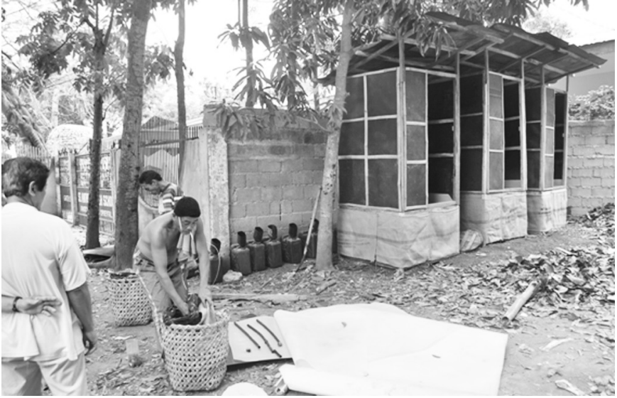
Photo 26: Installing the pre-fabricated units. Rattan basket is used for feces collection. Eco-Pees or male urinals lined at the side of the concrete fence.
