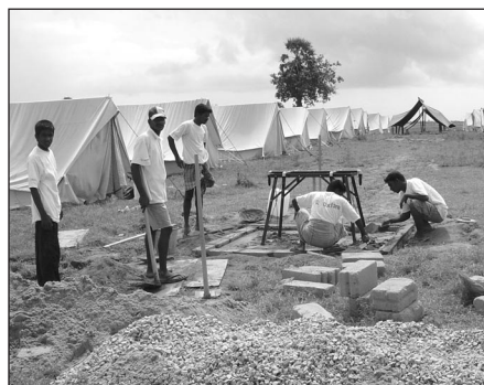
An Oxfam team installs a water distribution point in a Sri Lanka IDP camp
