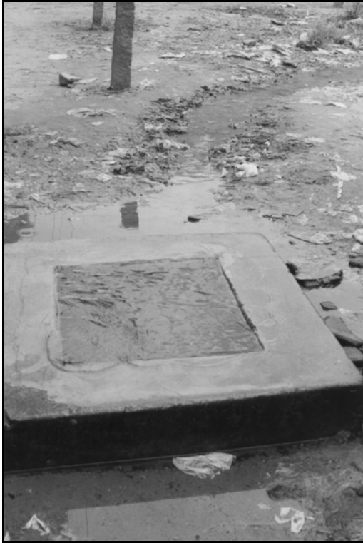
Figure 15: Open Aeration Tank: Overflowing and Surrounded by Solid Waste, Sillamarathupatti
