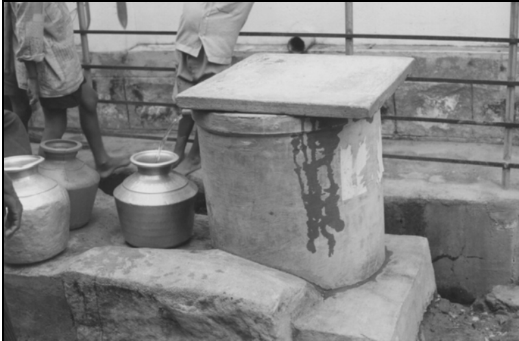
Figure 6: Closed Aeration Tank, Sillamarathupatti
