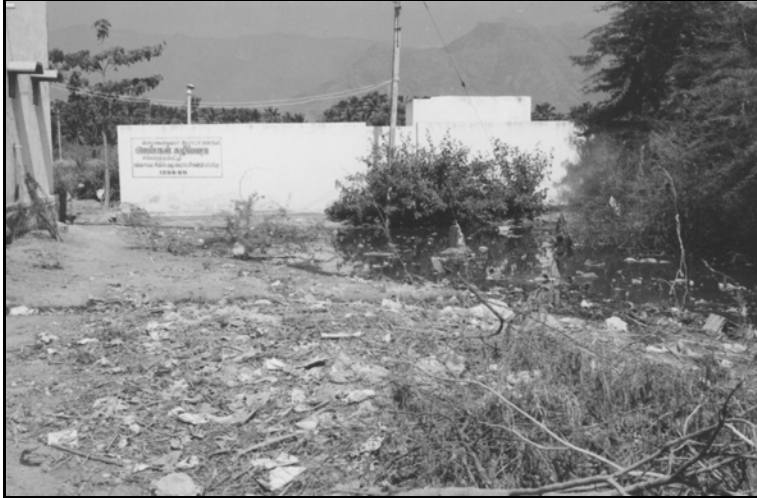
Figure 9: Non-functioning Women's Latrine, Northeast Scheduled Caste Colony, Sillamarathupatti
