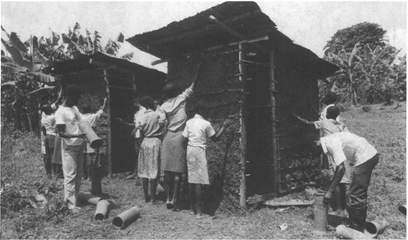
The new vent-pipes are inspected by the builders, and the latrines by the rest of the community.
