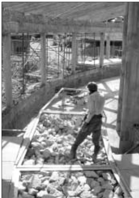
Installation of thermal rock stores at Harare International School in Zimbabwe: supply air is drawn through these cages from left to right (note deep solar shading created by extension of roof as veranda) (©ARUP/Mike Rainbow)
