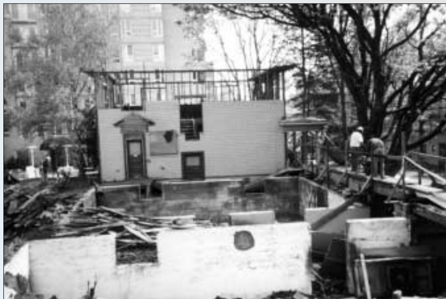
Progress in deconstruction of one of several 100-year-old houses in Portland, Oregon, by a non-profit company
