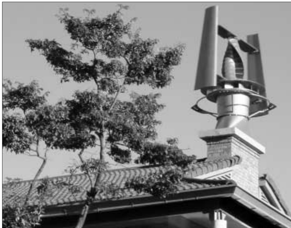
Turbine-type wind cowl on the roof of the Harare International School (©ARUP/Mike Rainbow)
