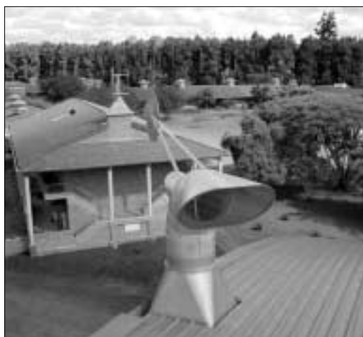
Wind-powered ventilation cowls on roof of PE hall at Harare International School (©ARUP/Mike Rainbow)
