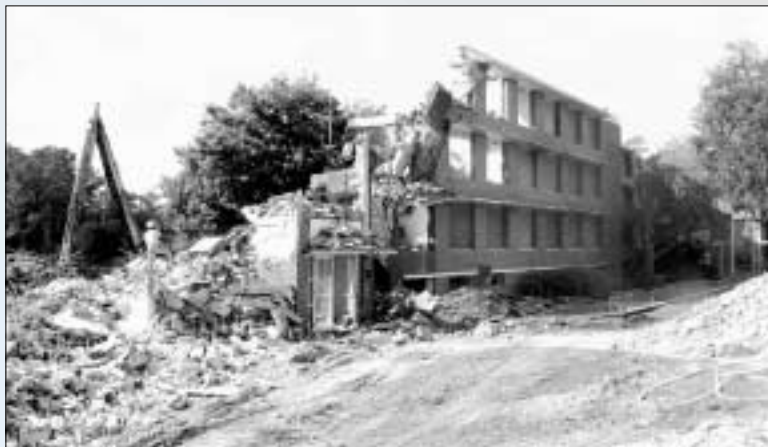
Demolition of Hume Hall, University of Florida, demonstrates a lack of capacity for recovering potentially valuable brick due to inadequate foresight in design and planning
