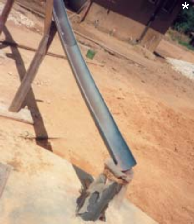
Figure 5-14: Closed up view of a connecting pipe made of half-cut PVC pipe collecting water from the gutter outlet to the tank inlet. The tank inlet is covered with a piece of nylon net to keep away the mosquitoes.
