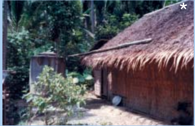
Figure 5-9: Even a thatch roof can be used as the catchment for rainwater collection. A half-cut PVC pipe or bamboo is fixed on the thatch roof as a gutter to collect rainwater into a tank.
