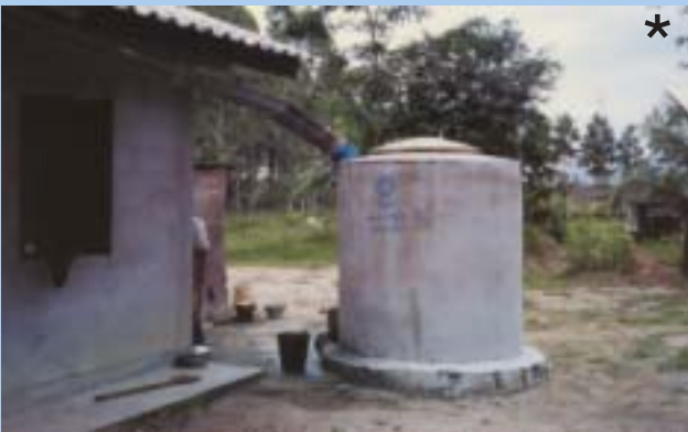
Figure 5-10: Gravalised sheet bent into "U" shape and fixed under the roof serves dual functions as rain gutter and connecting pipe to the tank.
