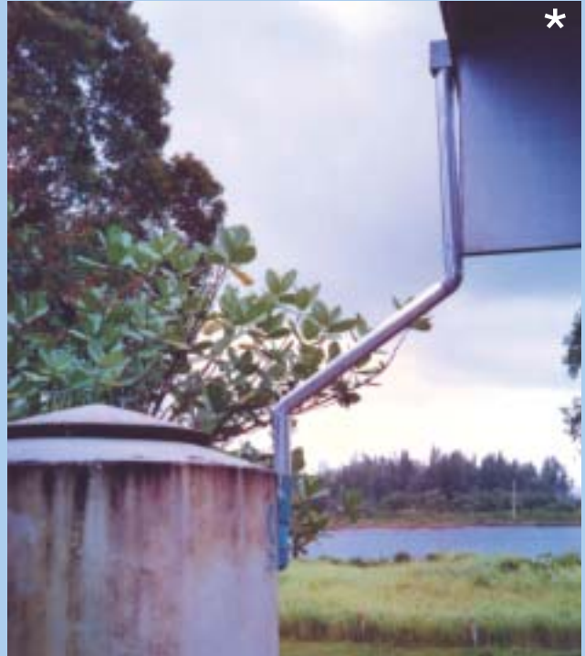
Figure 5-15: A gravelled pipe is fixed as the connecting pipe between the gutter outlet and the tank inlet.
