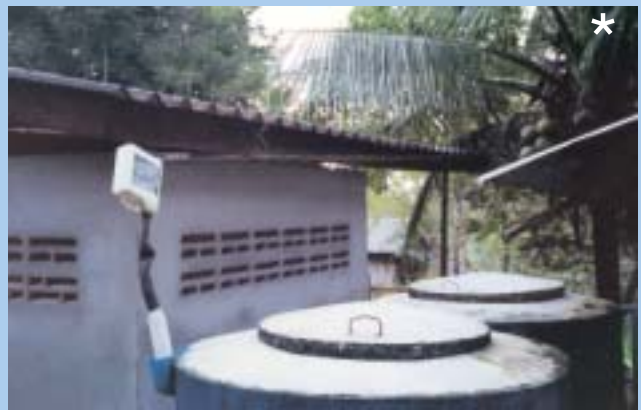
Figure 5-7: A plastic bottle is used instead of a funnel and fixed onto the connecting pipe inserted into the inlet of the tank.
