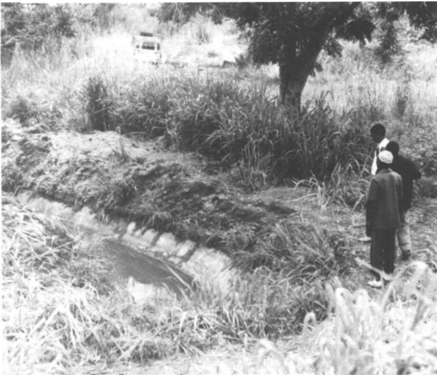
A secure livelihood for irrigators encourages reliable maintenance and better water and land management.
