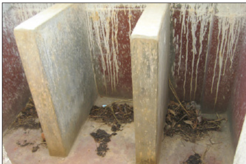
School toilets - built with public money but inaccessible to the children.
