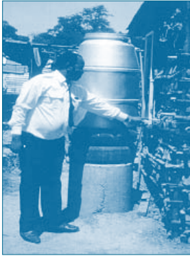
Outside view of ground tank
