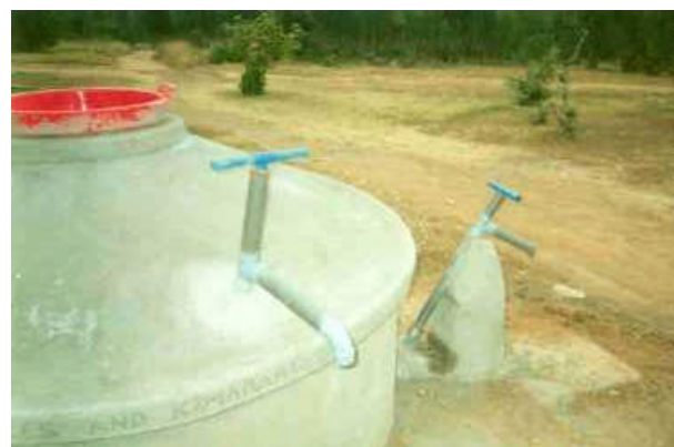
Figure 4 The DTU (left) and the Tamana handpumps fitted to a partially below ground tank
