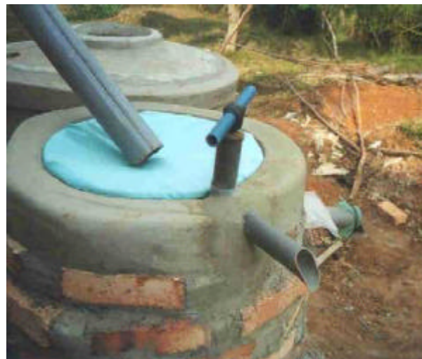
Figure 2 A Harold pump cemented into a plastic tube tank at Kyera Farm
