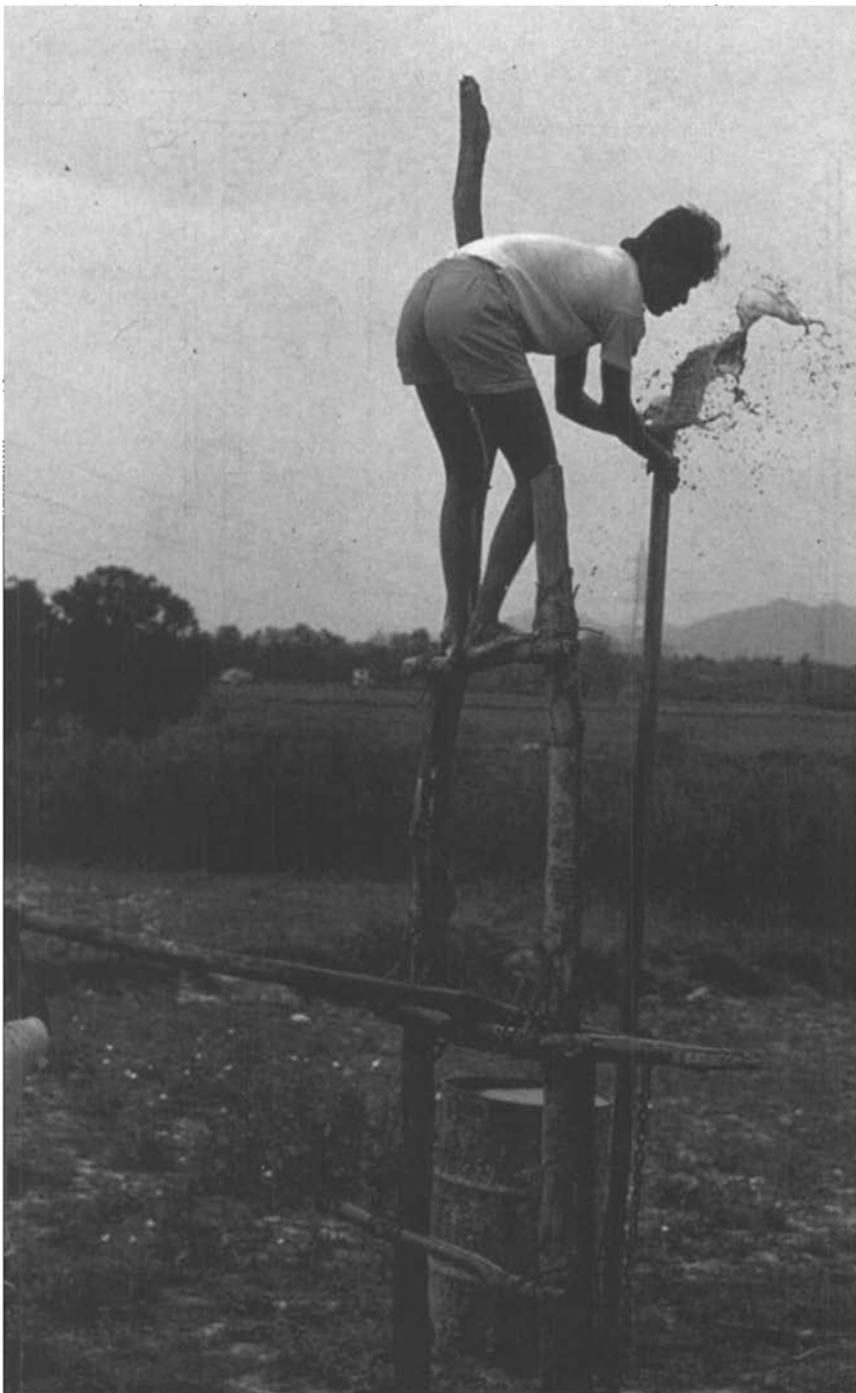
Water and mud squirts out of the top of the boring pipe on its down-stroke.
