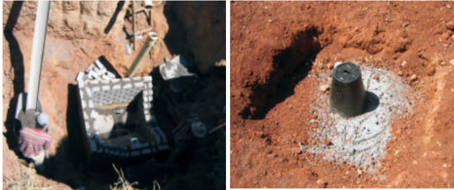
Example of manhole for gravity systems (left) and inspection pipe for vacuum systems (right) in Shoshong
