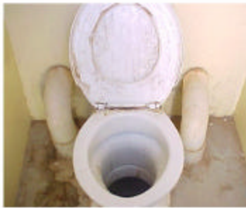
Enviroloo at the KDC offices
