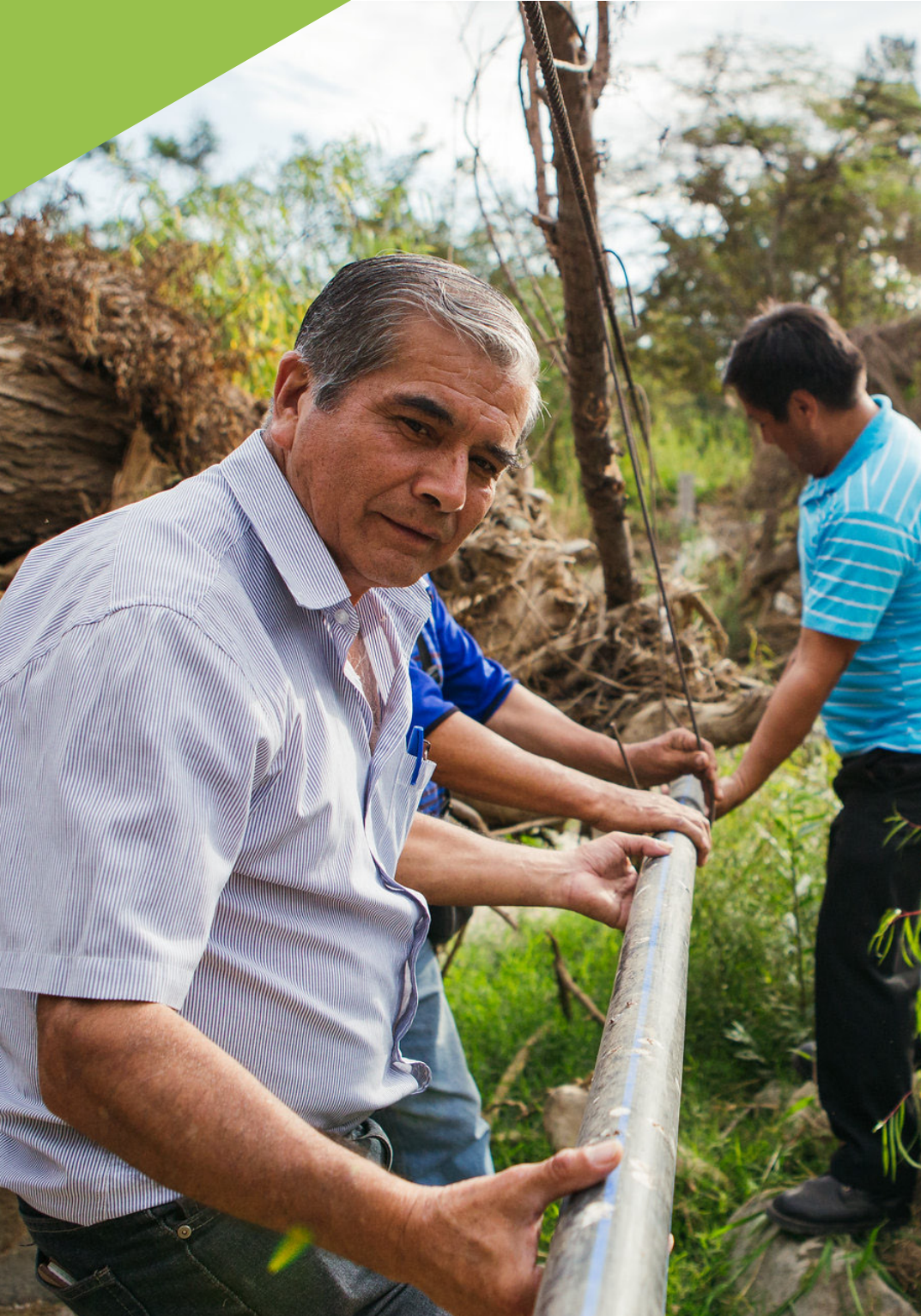
Technicians fitting a pipe in Pampas de San Isidro, Cascas, Perú (Water for People)
