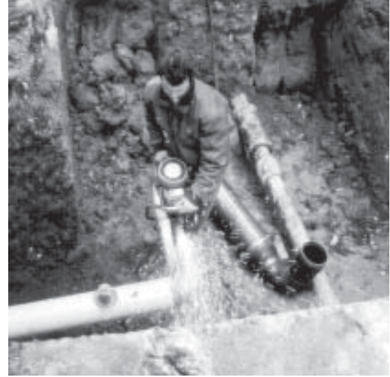
Often, working on the gas network is combined with renewing the water distribution network.
