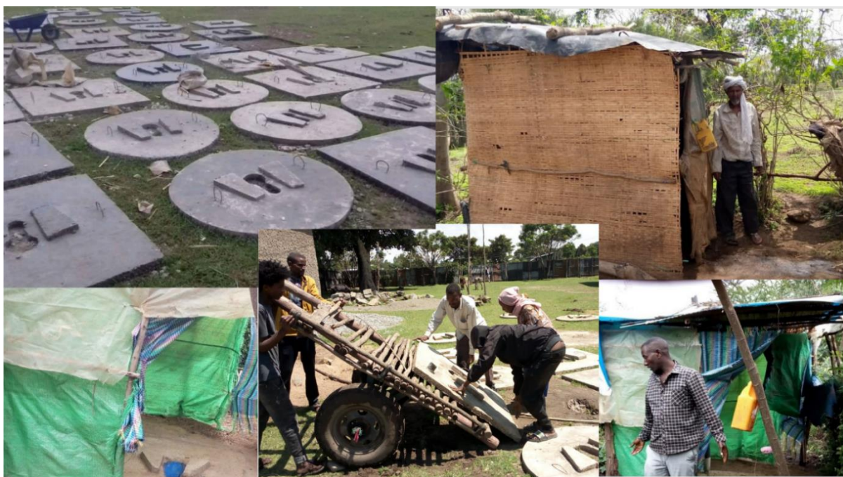
Figure 3: Production and distribution of latrine slabs and constructed improved household latrines. Photo credit: Amref Health Africa
