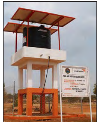
Solar powered mechanised borehole in Kenyasi No. 2
