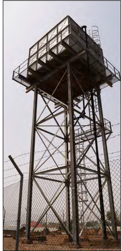
Overhead tank at Bongo Soe provides water to 6,000 people
