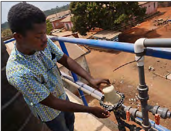
Martin Agyepong from Safe Water Network, checks a filter on the water tower at Wamahinso
