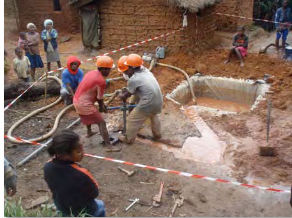
Teams from the local enterprise BushProof installing a borehole using the EMS manual drilling technique
