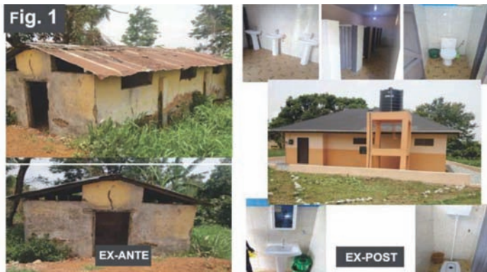
The construction of Abetifi Presby Primary & JHS school 14-seater WC toilet with hand washing facilities.
