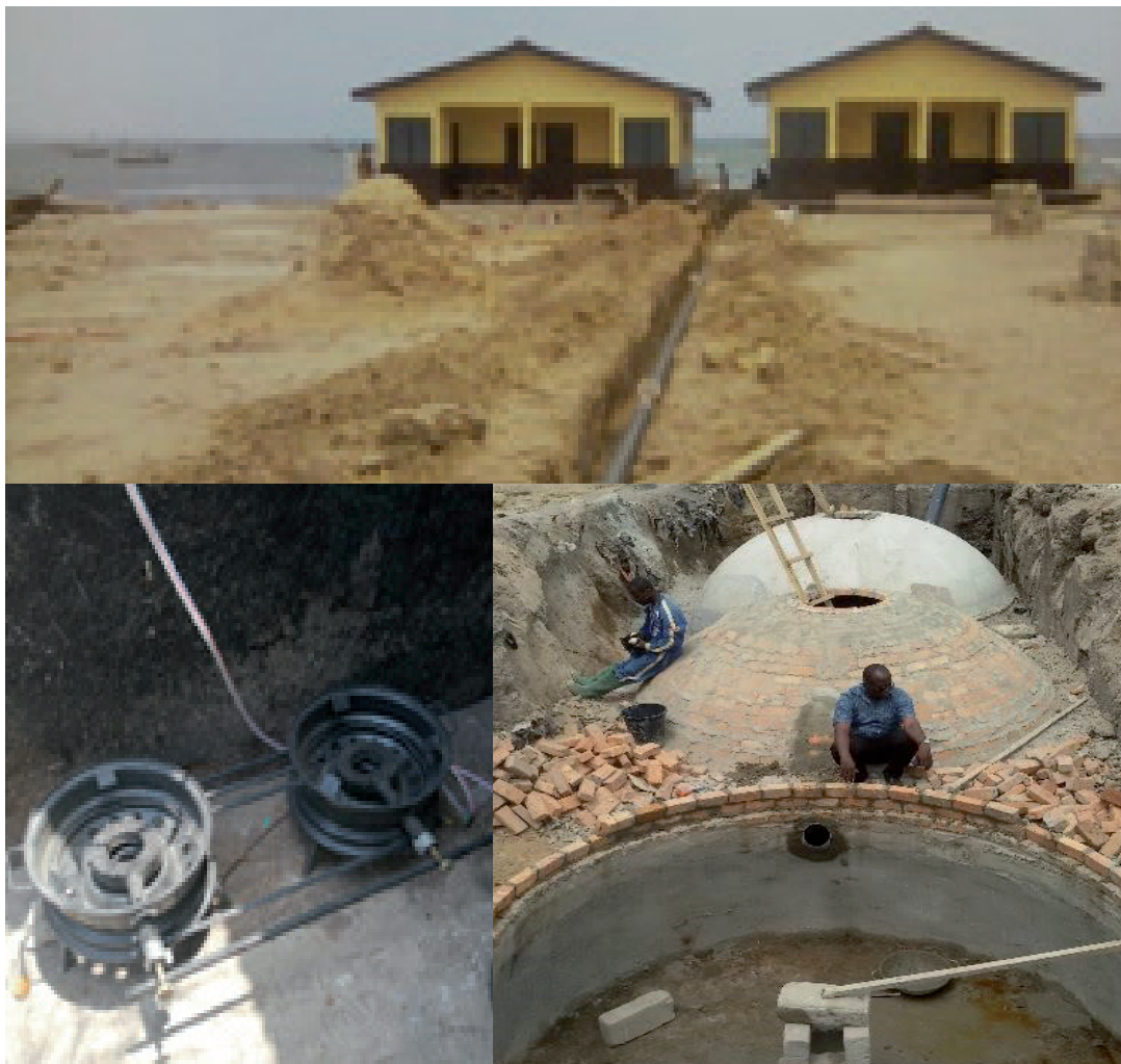
Gas line back to prisons (top), gas used at prisons kitchen (bottom left) and construction of biogas toilets (bottom right)..
